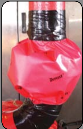
Offshore Platform Fire Water Line
