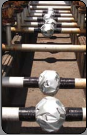
Inland Terminal Oil Lines
