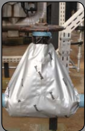
Coastal Terminal Oil line with Gate Valve
