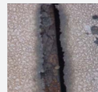
Corrosion at a support beam
